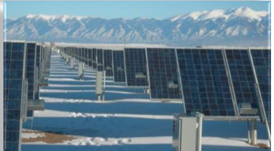
Alamosa PV System, Alamosa, CO
